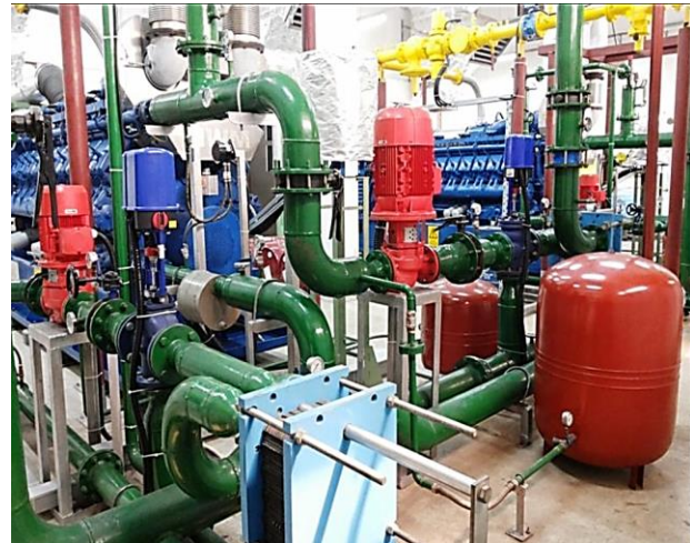
Gas Genset Auxiliary Piping
