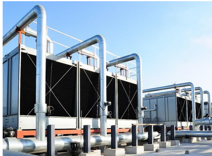
Cooling Water System
